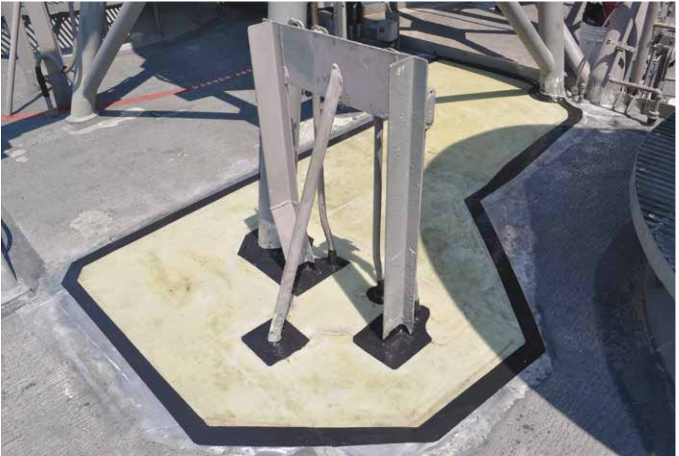
A composite patch repairs a CG-47 class ship's cracked aluminum superstructure. If successful, it will save $30 million over 5 years.
